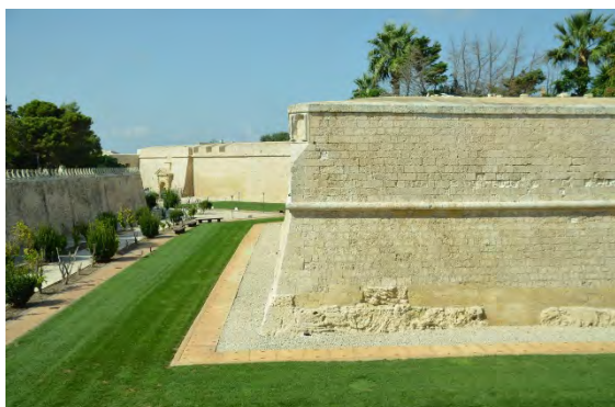
Fig. 32: View into the moat of Mdina with the Greek gate visible in the background.
