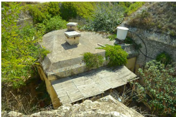
Fig. 36: The over-concreted trench caponier on the left side of the Tas-Silġ fort.
