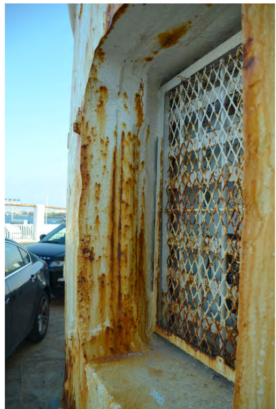
Fig. 15: A sandwich construction of the Gibraltar shield also in Malta at Sliema Fort.
